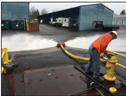
30-inch – Fire Hydrants
